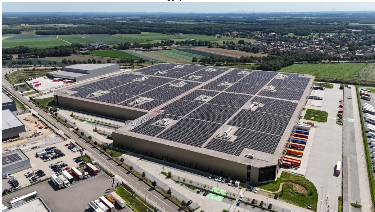
Legend: Sunrock solar power installation on a logistics building Photo credit: Sunrock
